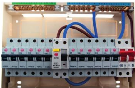
▲ Figure 6.2 Circuit breakers in a consumer unit
